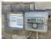
Typical irrigation control box
