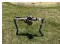
Typical irrigation backflow
